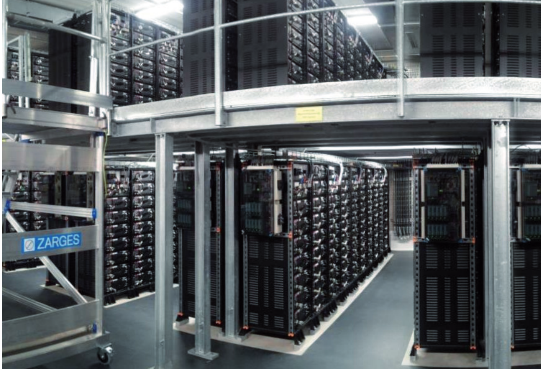
Figure 3.3.3.2.5: Interior view of the first commercial battery power station in Germany. The 5 MW lithium-ion facility has the equivalent reserve capacity potential of a conventional 50 MW turbine. | Source: WEMAG.
