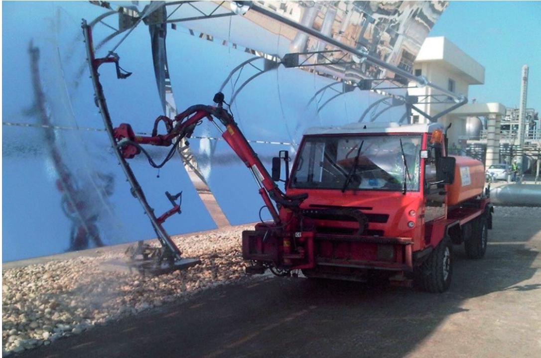
Figure 3.1.2.2: Cleaning a solar trough power plant, Kuraymat, Egypt. | Source: Gerhard Hofmann, Agentur Zukunft.
