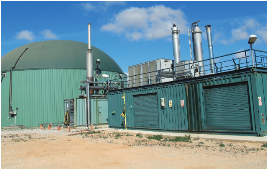
Figure 3.1.5.2: A biogas-producing anaerobic digestion plant. | Source: RENAC.
