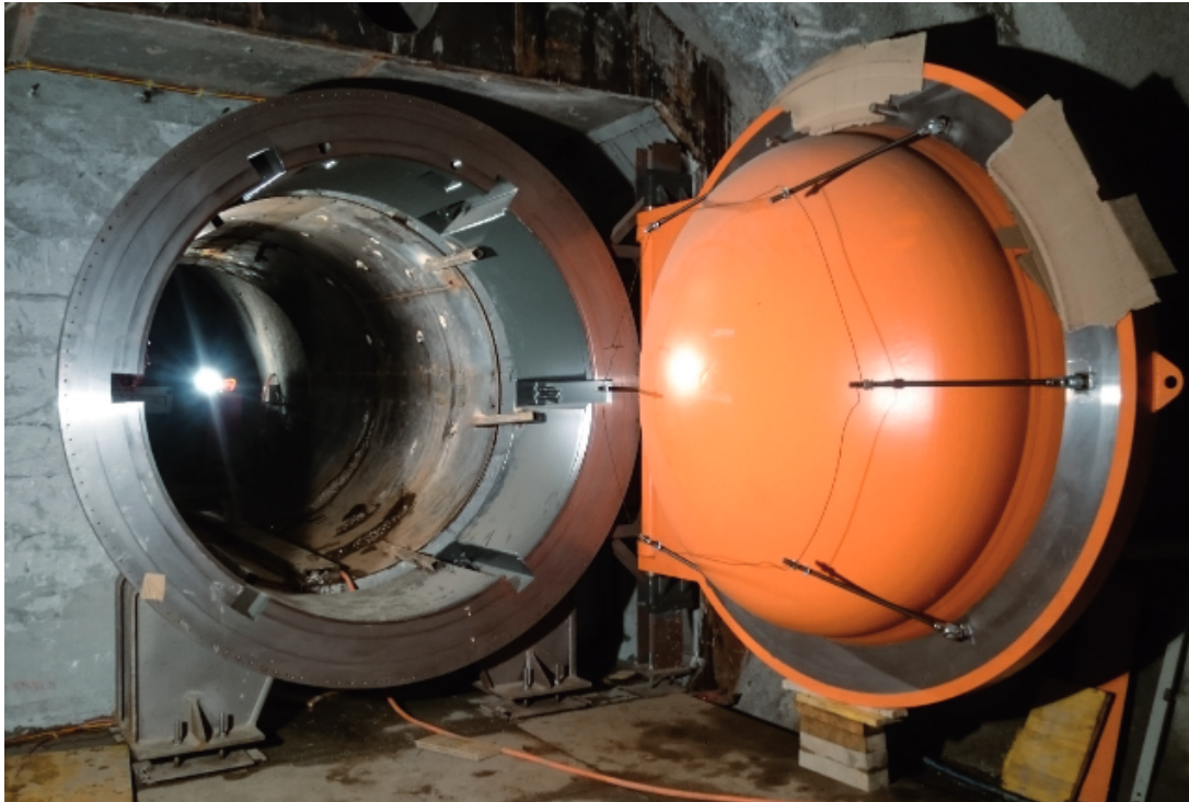
Figure 3.3.1.3.3: Rock cavern pressure vessel access door. | Source: ALACAES SA.
